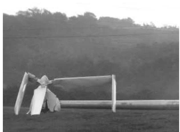
Downed Wind Turbine at Teignmouth
